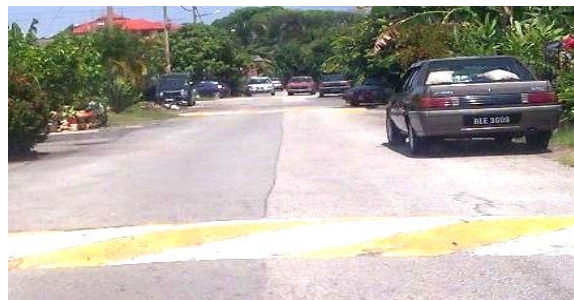
Figure 3. Surface condition of the residential area road used in this study.
